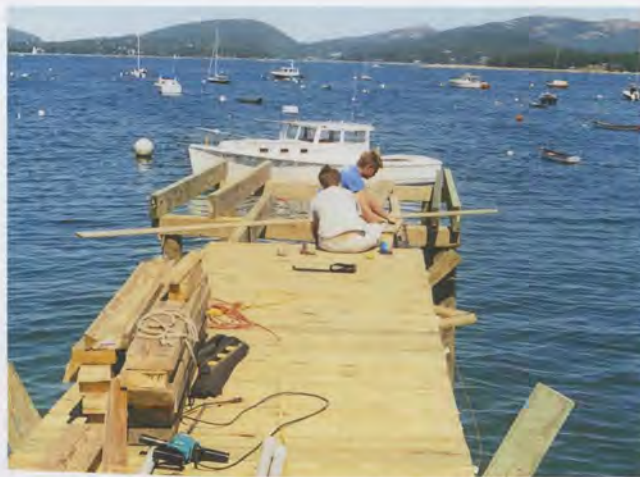
August 2002—Martha and Josh built a 110-foot dock for the boatyard. It took their entire summer vacation to build the dock, main float, and two finger floats.
